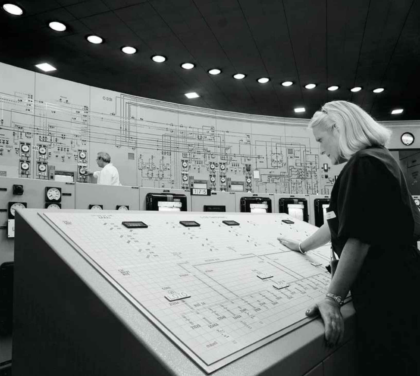
Judy Smith verifies power distribution during a switching operation while Clint Dixon monitors equipment in the central control facility.
