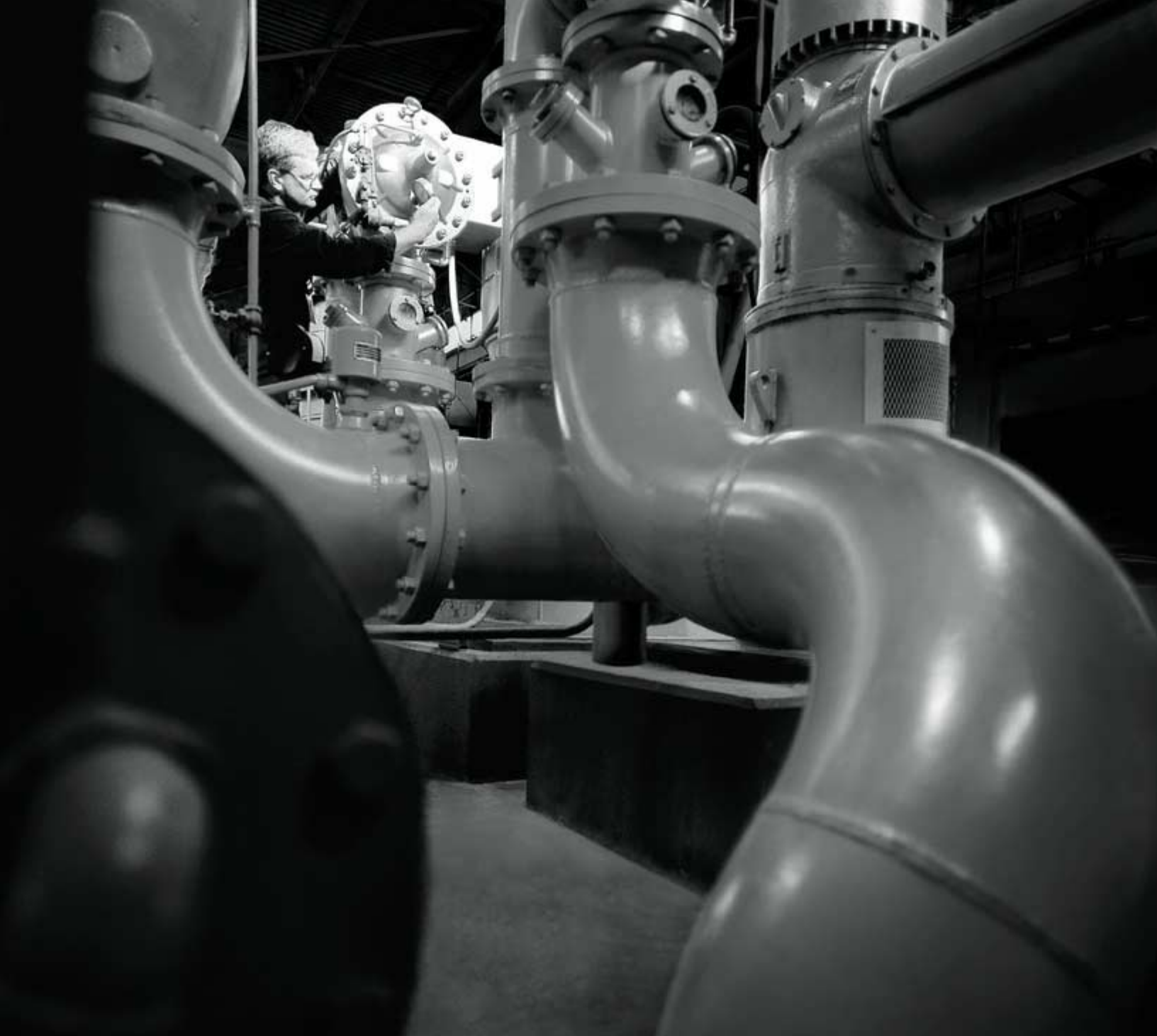
In the pump house, Kevin Lindsey monitors discharge pressure on pumps that control the firewater systems in the plant.
