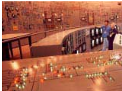
Nerve center – Paducah control room.
